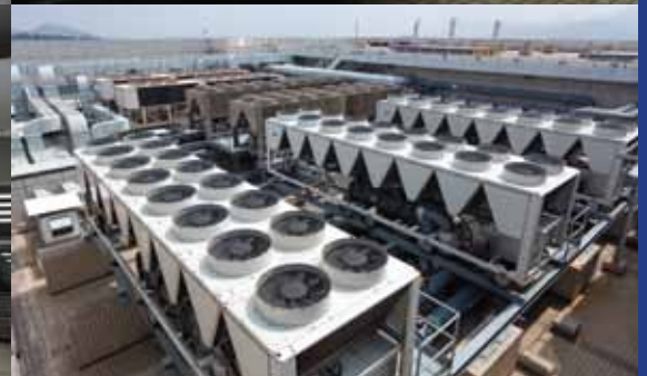
Air-Cooled Chillers (Standby)
