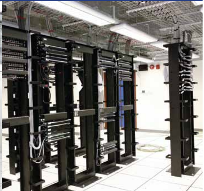
Core Switch Room
