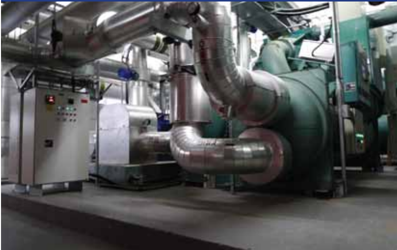
Water Cooled Chillers (Duty)
