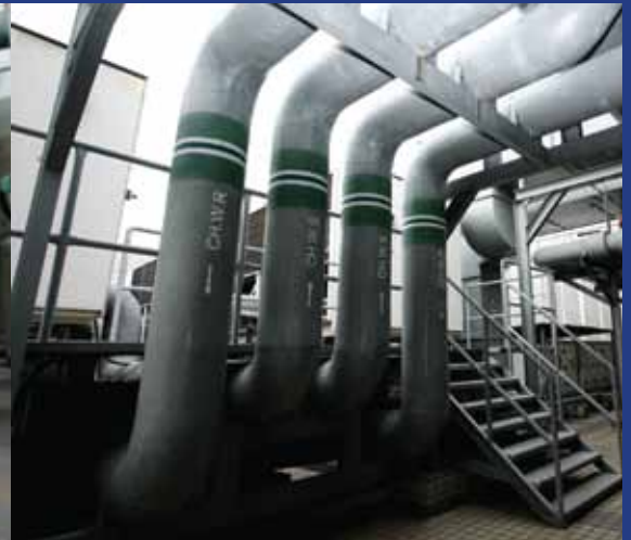
Dual Chilled Water Distribution Rings
