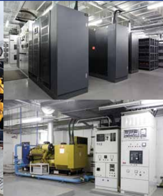
Centralized 2N UPS
